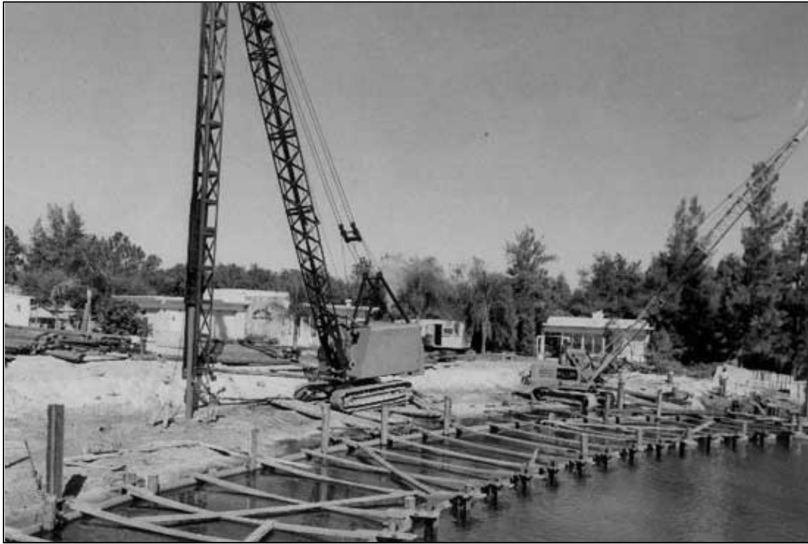
Figure 2-5. Construction of the current underwater theater in 1959. Courtesy Florida State Parks ( http://www.floridastateparks.org/history/parkhistory.cfm?parkid=196 ).
