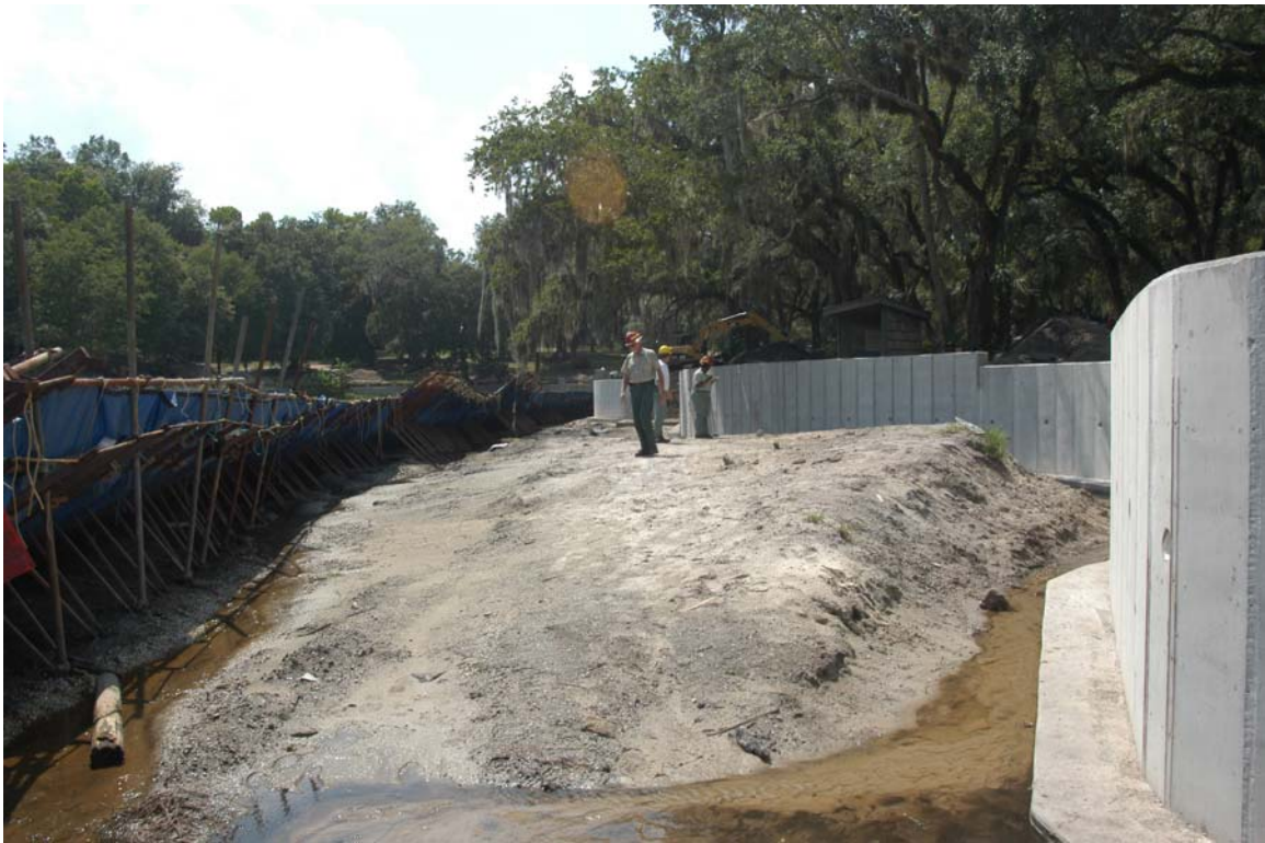
Figure 1-5. View facing northwest of the exposed near-shore deposit between the coffer dam (left) and the concrete bulkhead (right).
