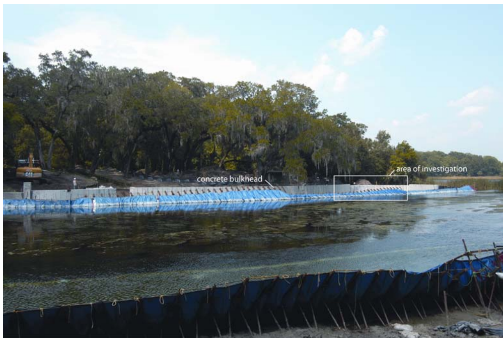
Figure 1-4. View of Salt Springs pool facing east, showing coffer dam (blue structure), placed concrete bulkhead, and area of archaeological investigations.
