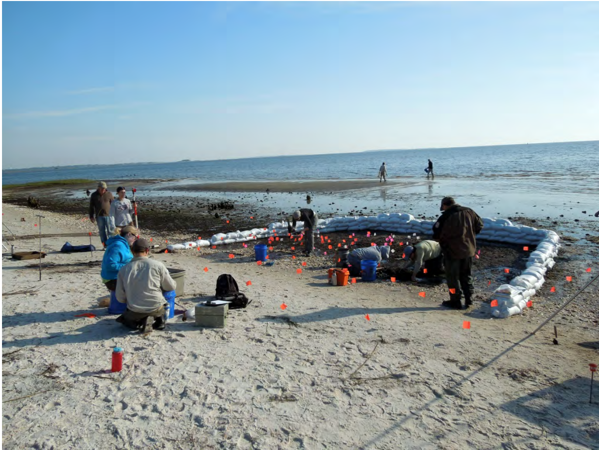
Figure 2-6. View facing south of the semi-circular berm of sand bags emplaced around human burials on the south shoreline of McClamory Key.
